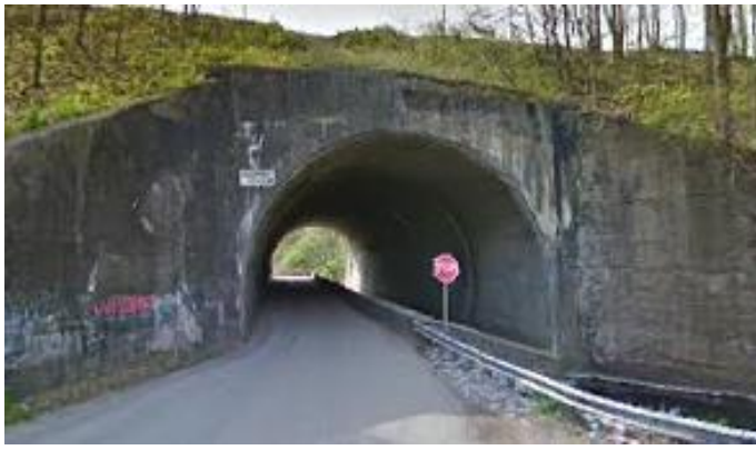
Corvette Tunnel with roadway in left half and Piney Fork Creek on right.
