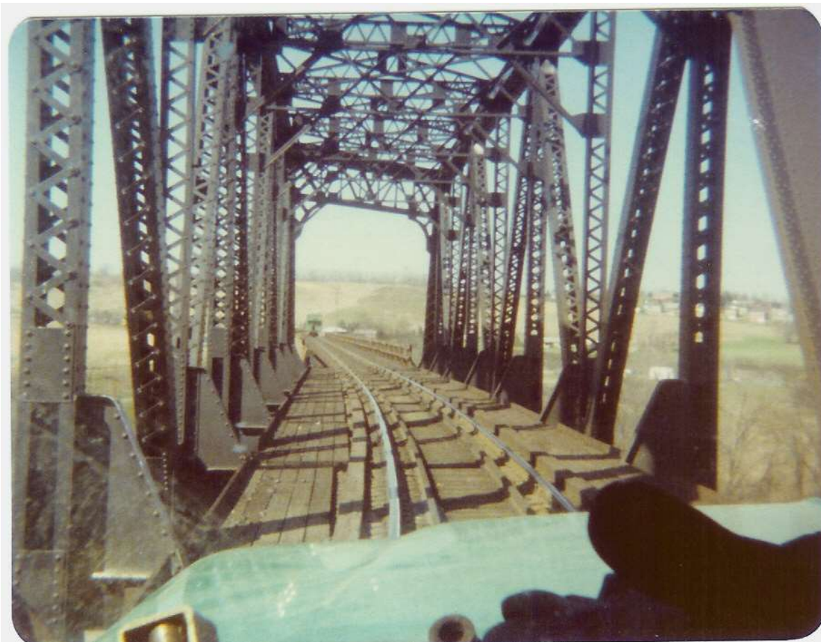
A view out the windshield of a track gang hi-rail truck as they transit the through-truss span of the McDonald Viaduct in 1976. The open framework supports a timber deck. Tim Sposato photo.
